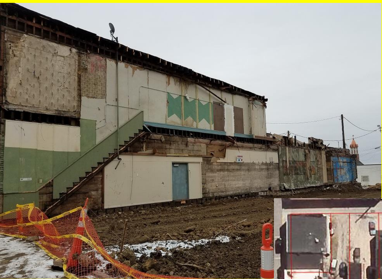
This owner's wall is not an exterior wall and the demo left him with a lot of exposure. Business has closed until further notice.
