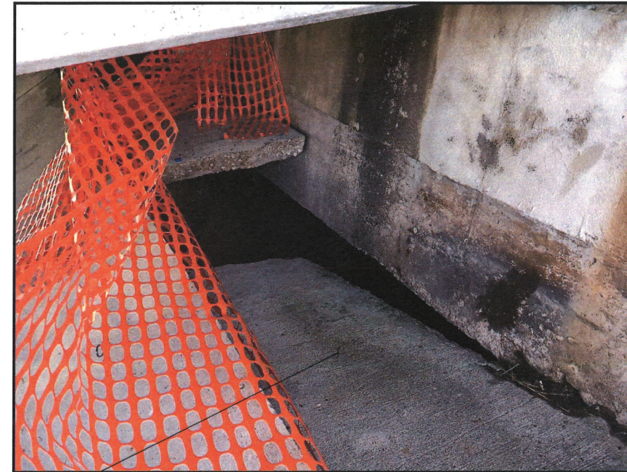
FAILED & UNDERMINED SLOPE PROTECTION PANELS
