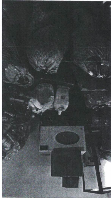
Apt 4 picture from first inspection indicating did not remove damaged materials and just plastered over.
