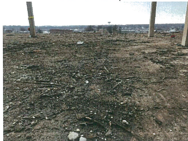
Fourth floor damage
