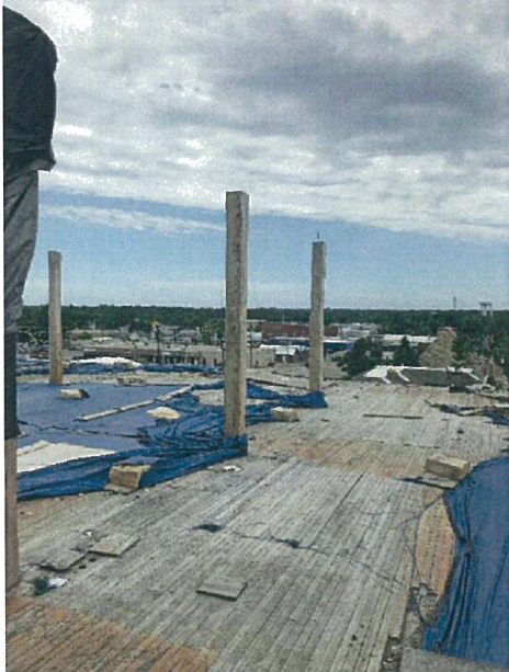
Fourth Floor damage detail
