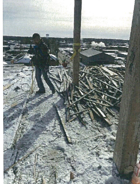
Fourth floor damage
