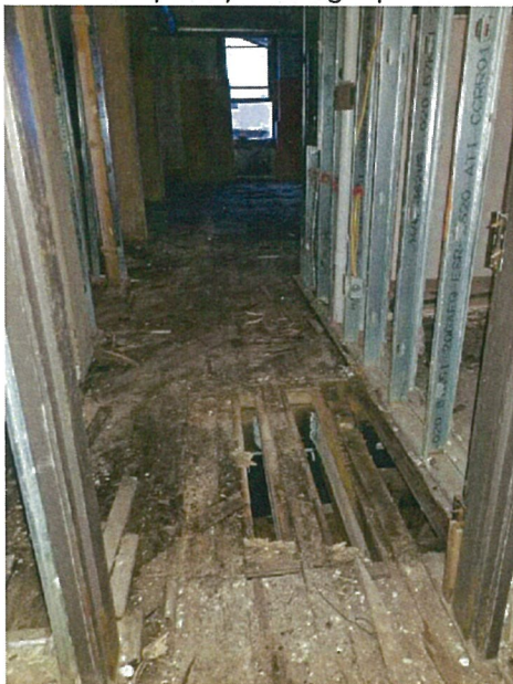
Flooring damage, lower floors
