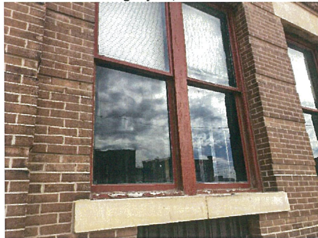
Fractured window panes
