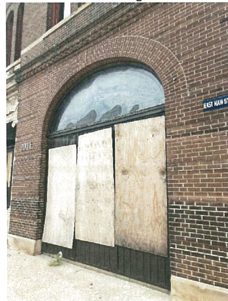
Window damage along Main Street
