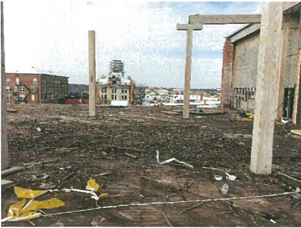
Fourth floor damage
