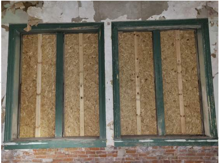
TYPICAL CONDITIONS AT BUILDING #6.
