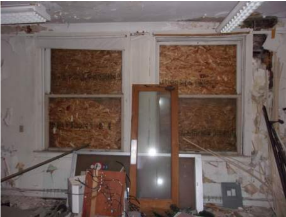
TYPICAL INTERIOR (2ND FLOOR) CONDITIONS AT BUILDINGS #2 AND #3.
