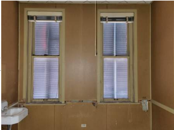
TYPICAL CONDITIONS AT BUILDING #7.
