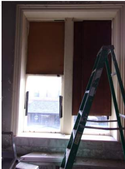
TYPICAL CONDITIONS AT BUILDING #5.
