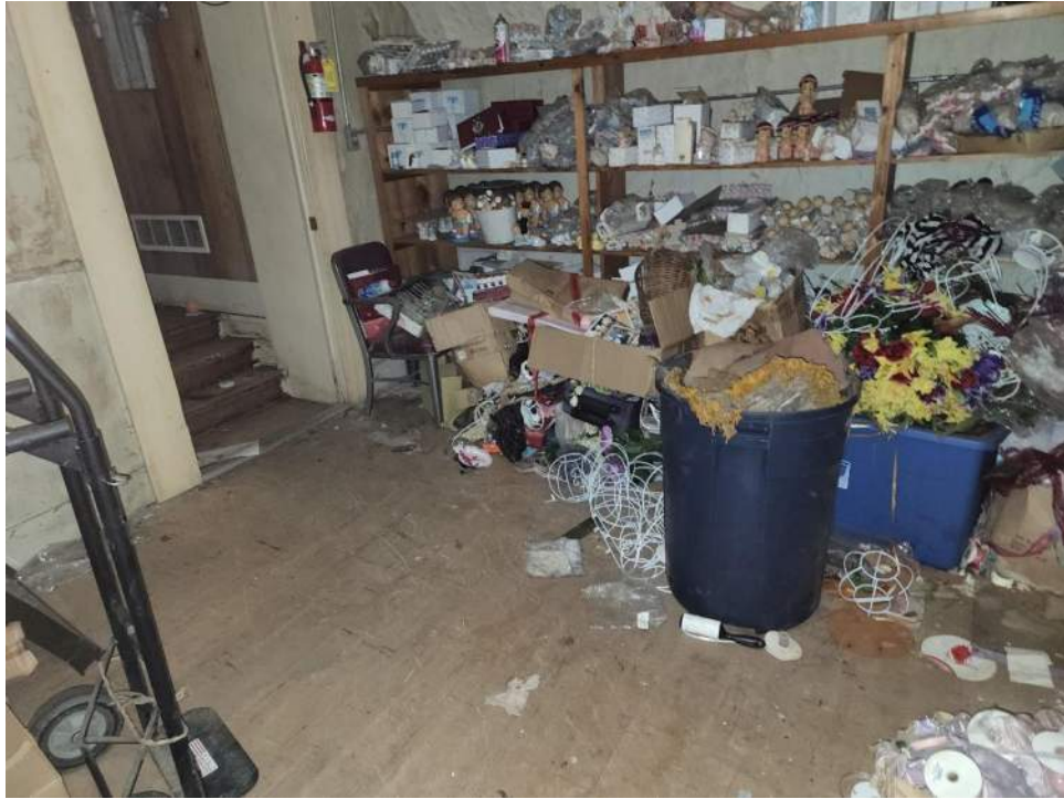
Property Photograph 7 – Debris in main room, 2 nd floor.
