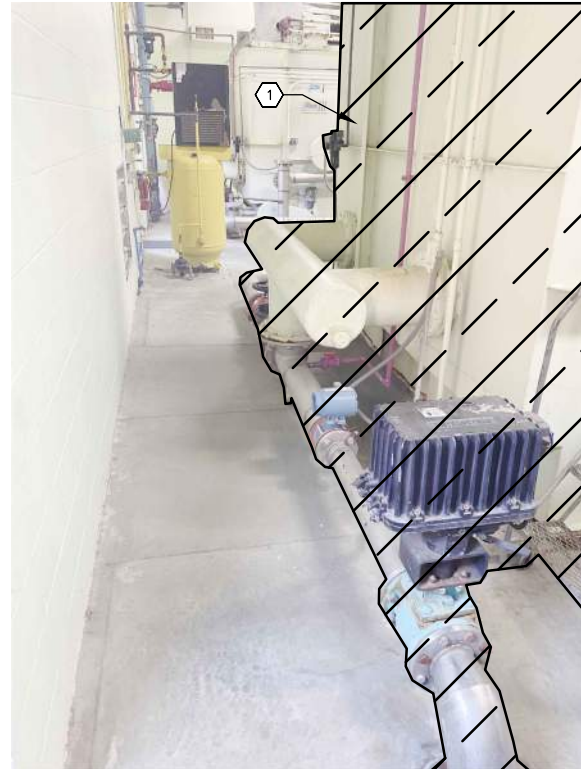
3 SOUTH DAF WEST SIDE PIPING FACING NORTH NTS
