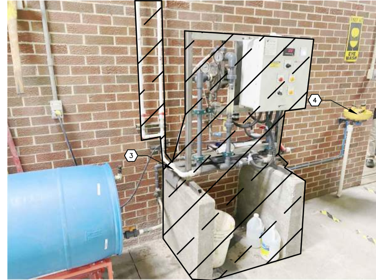
7 POLYMER FEED SKID FACING SOUTH SCALE: NTS
