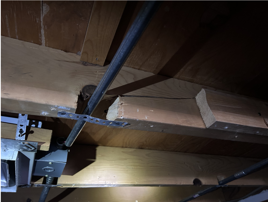
Figure 6 – View of typical notch in joist for conduit. Note split in joist due to notch.
