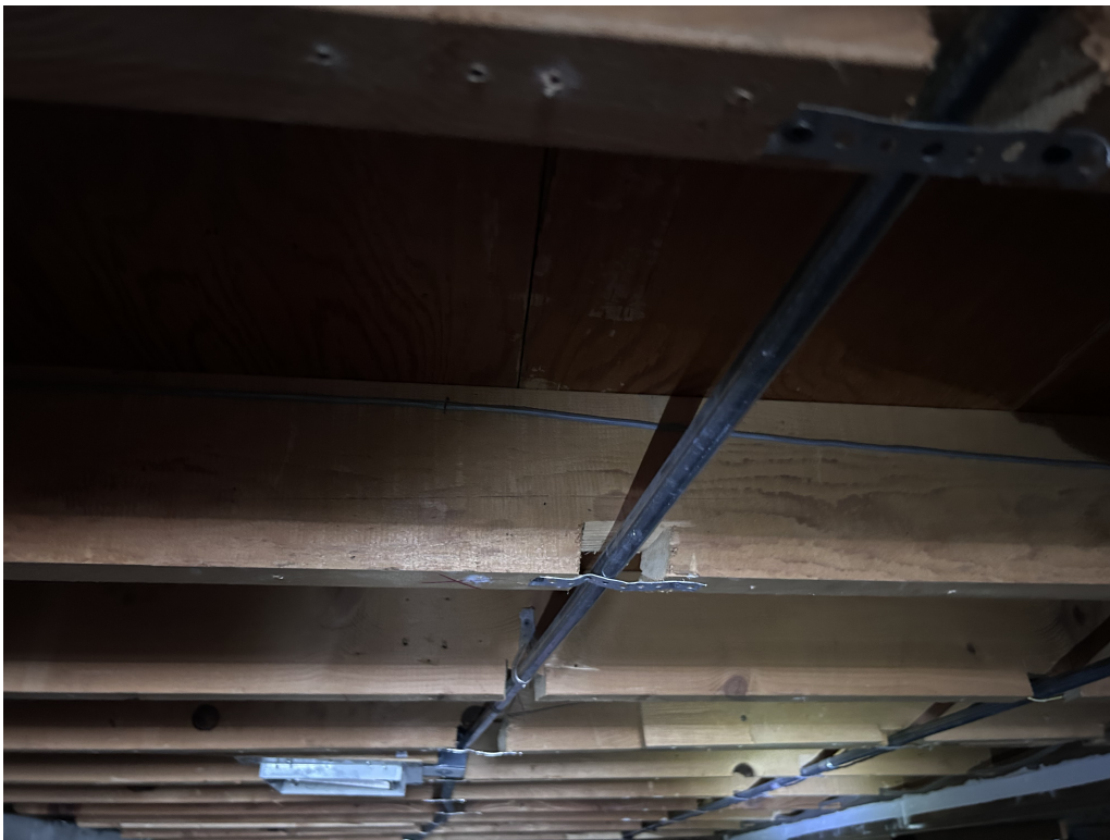
Figure 9 – View of multiple joists with notches.
