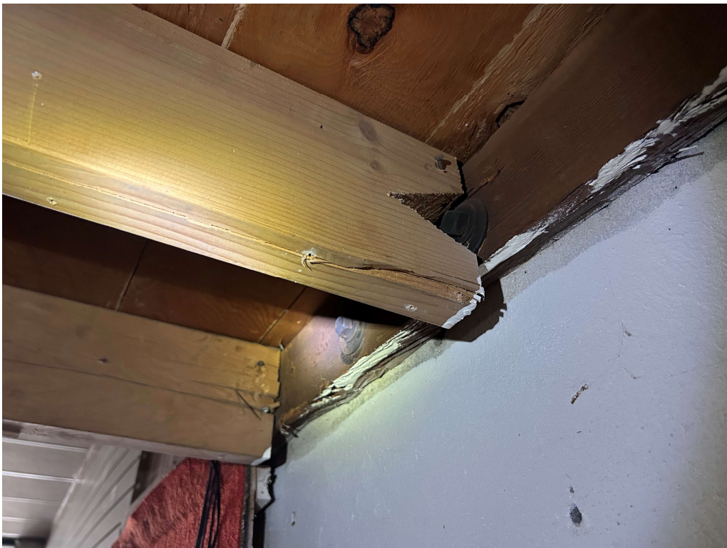
Figure 5 – View of typical floor joist notched to accommodate ledger bolt.
