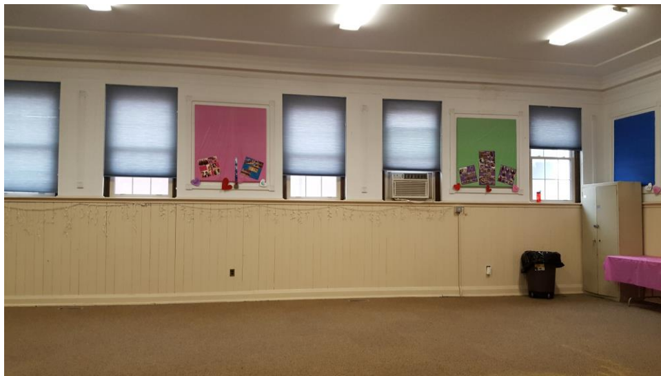
Figure 4: Blue Room showing window-mounted air conditioner
