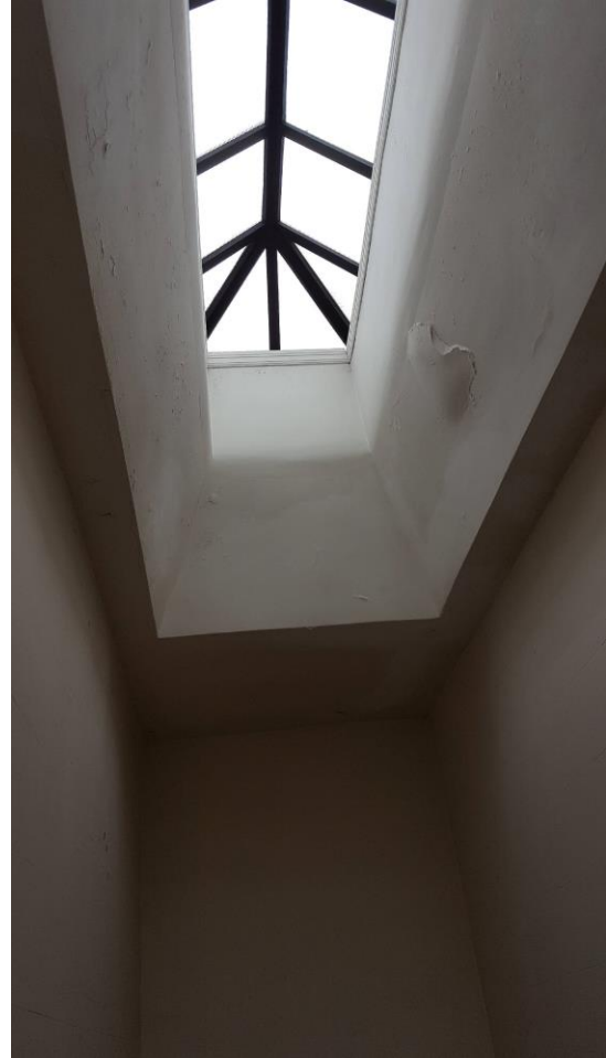
Figure 16: Water damage under skylight
