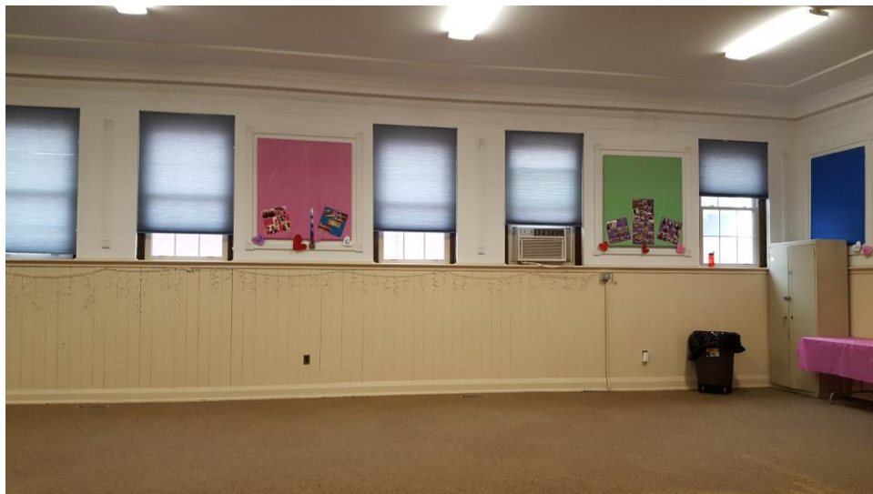
Figure 4: Blue Room showing window-mounted air conditioner
