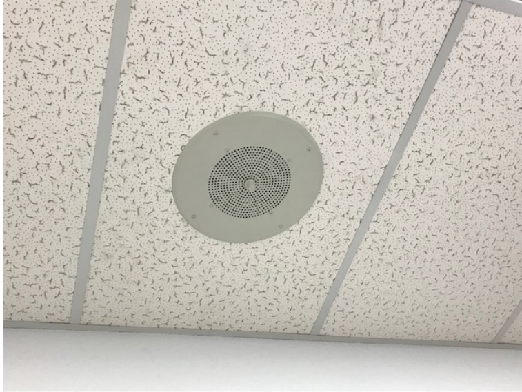
Portions of the station paging/alerting system being reused.
